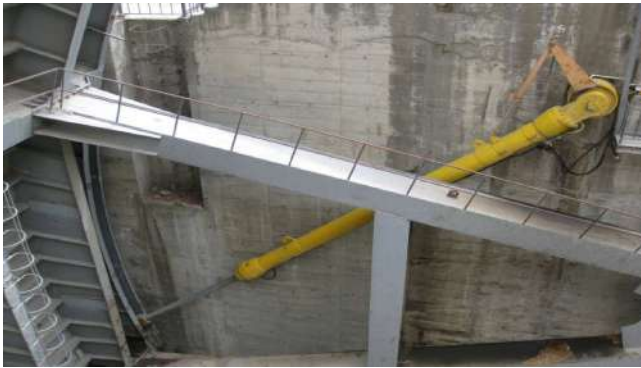
Hydraulic Cylinder - Radial Gate
